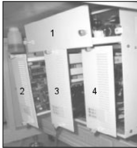
[C/B Rack Structure]
